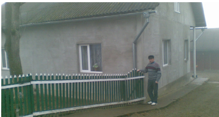
The house of the Ukrainian family from Velesniv before the reconstruction and after outer insulation and windows replacement.
